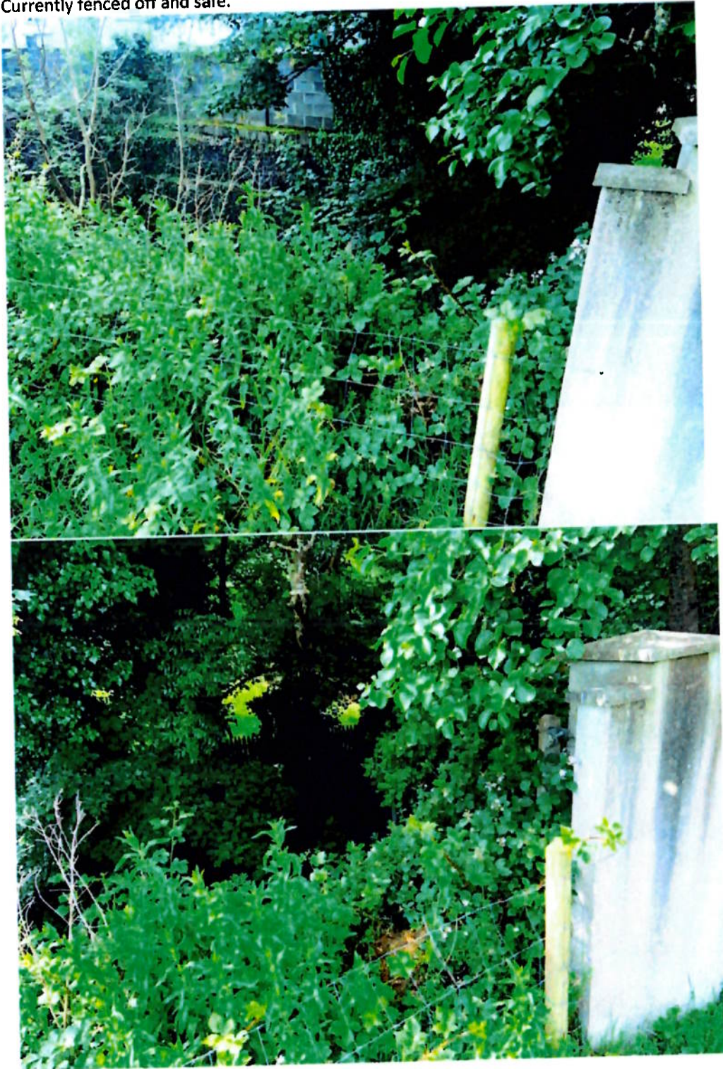
Photos E & F: 10 foot near vertical bank with walls at top. Downstream from culvert. Currently fenced off and safe.
